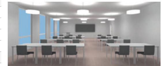
Classroom with 9 Milano LED luminaires
